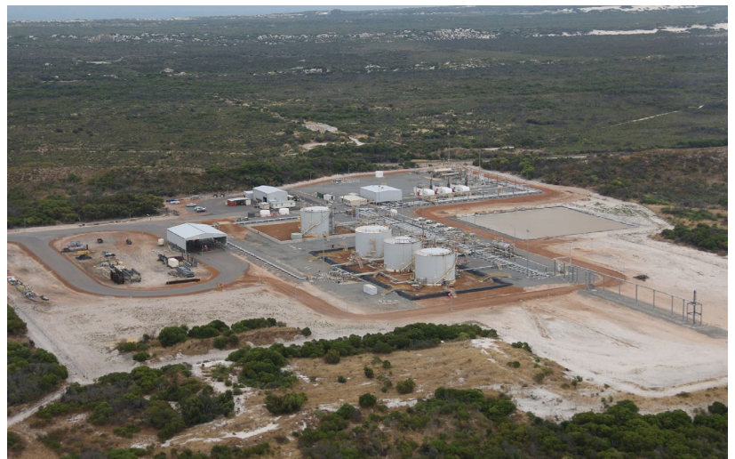
Arrowsmith Stabilisation Plant
