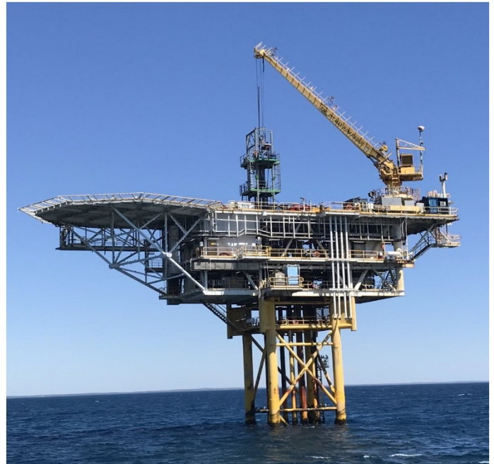
The recently commissioned Hydraulic Jacking Unit (HJU) at Cliff Head Alpha
