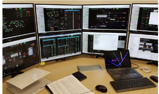
Testing of new Operations Centre in West Perth
