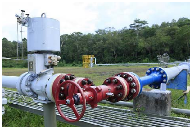
Figure 3: New adjustable choke installed on A-6
